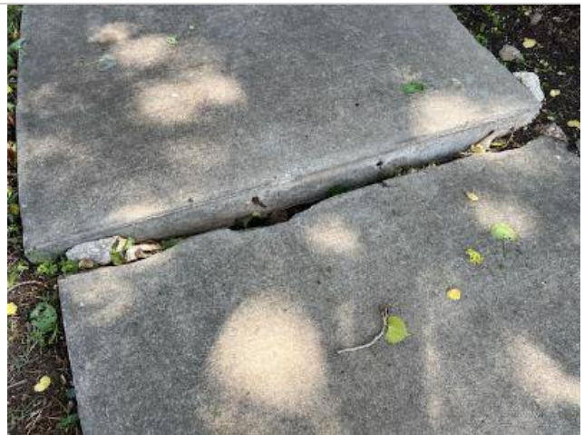
Concrete sidewalk trip hazards were observed in isolated locations
