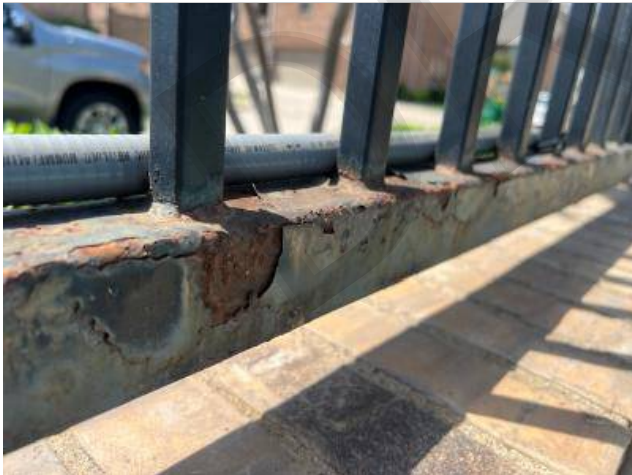
Pool Fencing, Deterioration noted in isolated areas.
