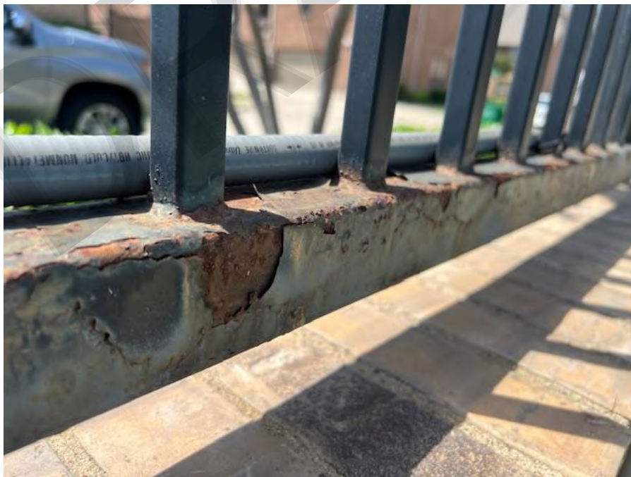
Pool Fencing, Deterioration noted in isolated areas.
